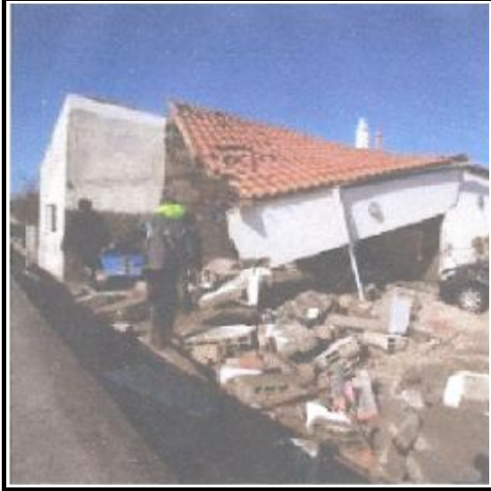
A cottage devastated in the storm.
