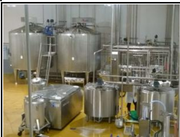
Some of the "State of the Art" stainless steel equipment at the Jersey Dairy. This photo, and the one on the previous page were taken by Robin Perchard.
